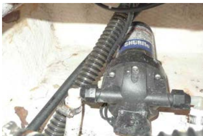
Shurflo Blaster raw water washdown pump. Shurflo livewell supply pump Rule 750 GPH cartridge type livewell drain pump. All smoothbore hoses & anti-siphon loops at discharges.
