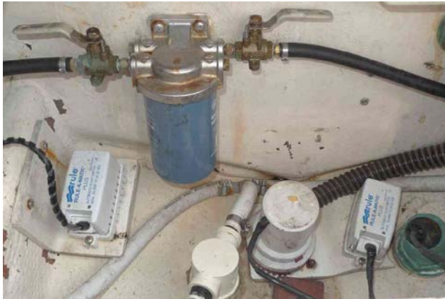
Left to right: High water alarm float switch Yamaha 10 Micron fuel filter & shut offs Raw water washdown inlet strainer Rule 2000 bilge pump & float switch Airmar 600KW 50/200 Hz 20° tilted element transducer
